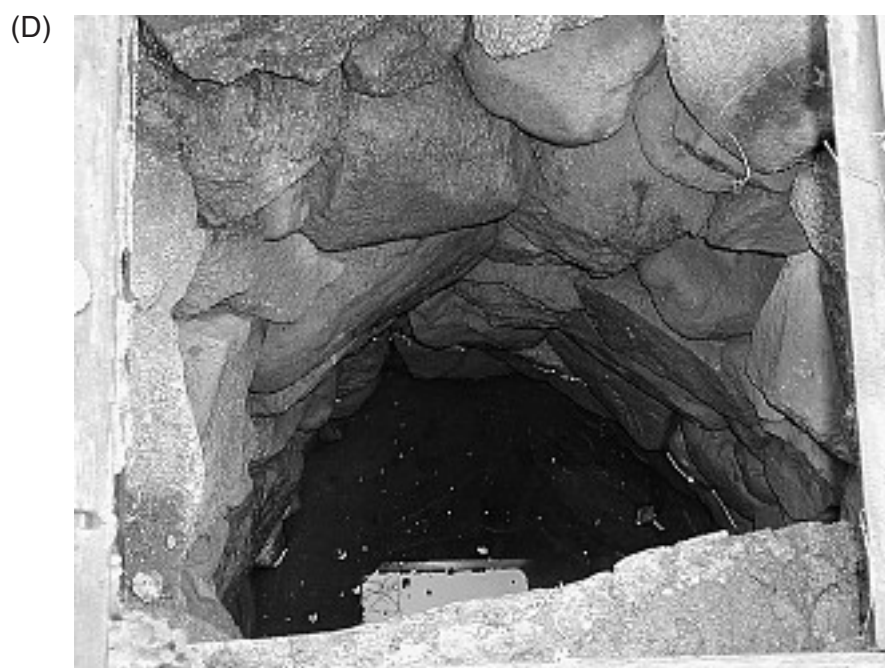
Fig. 35. Types of wells sampled in 1990: A) dug well, B) bedrock well C) spring D) stone lined well.
